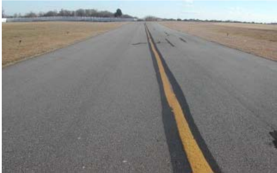
Figure A2-38 Taxiway C with Low Severity Cracking
