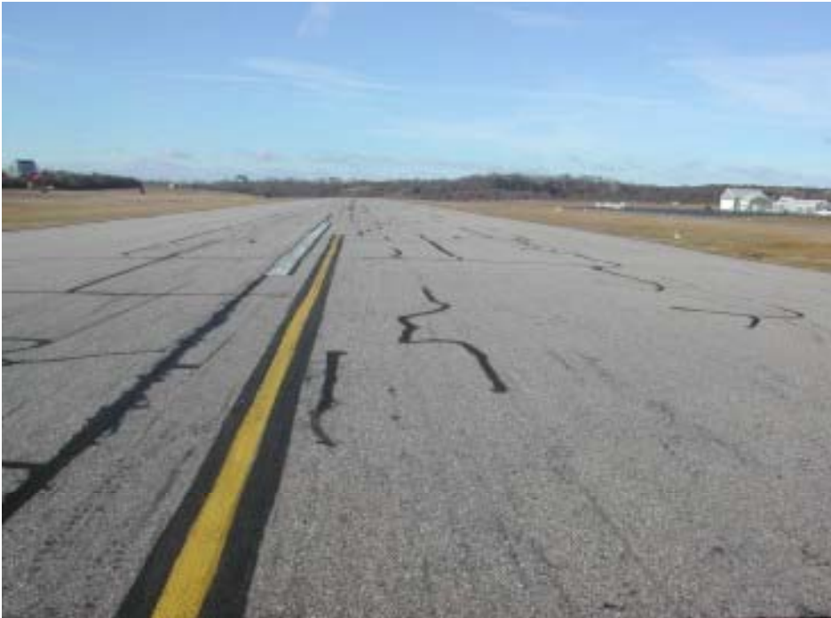
Figure A2-39 Runway 10-28 with High Severity Cracking
