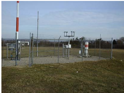
Figure 4-1 AWOS Weather Station
